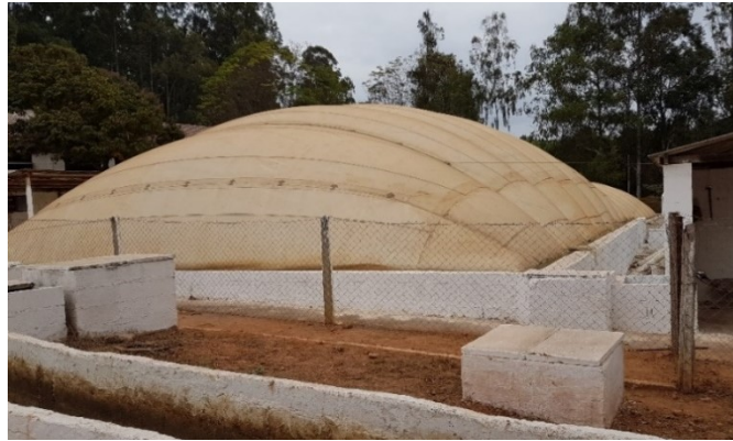
Figure 7 - Tubular anaerobic digester of the Nursery Site.
