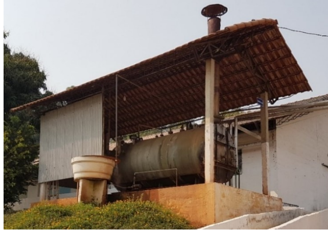
Figure 8 - Tubular biogas boiler.
